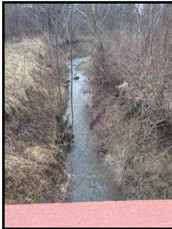
Figure 16: Looking upstream, inlet to Upper Lake Dam, Hudson, Summit County, the creek is incised here with eroding banks.
